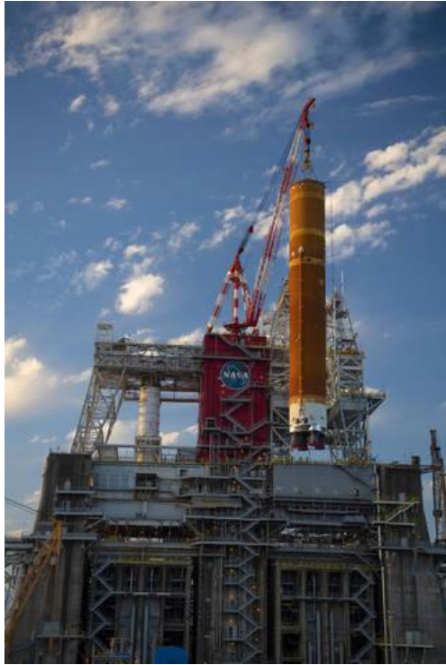
Core Stage being lifted into Stennis Space Center test stand for Green Run Test Firing
